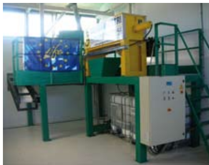
Decentralised oil press installed for the VOICE project © CREAR
